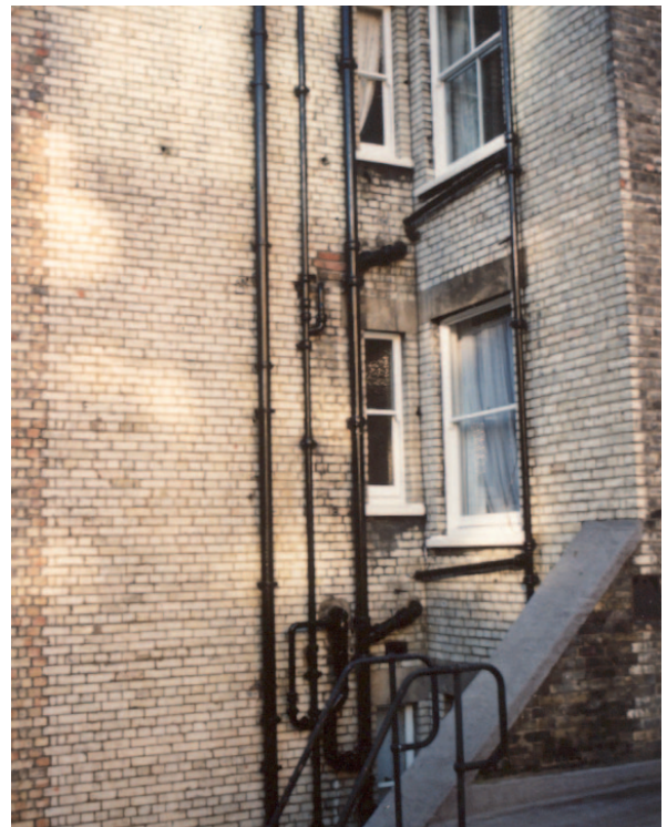
Figure 9: White walls require regular maintenance or their reflectance will deteriorate, as shown here
