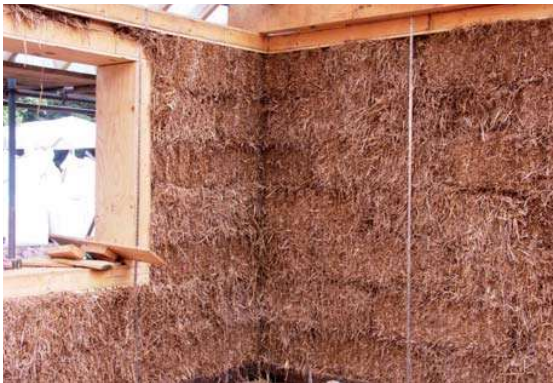
Figure 8: A completed wall with straps connecting the wall plate to the base (Courtesy of Mike Beckett/Collins & Beckett)
