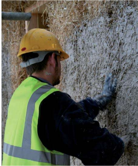
Figure 9: Vapour-permeable render being applied to exterior of straw bale surface (Courtesy of Mike Beckett/Collins & Beckett)
